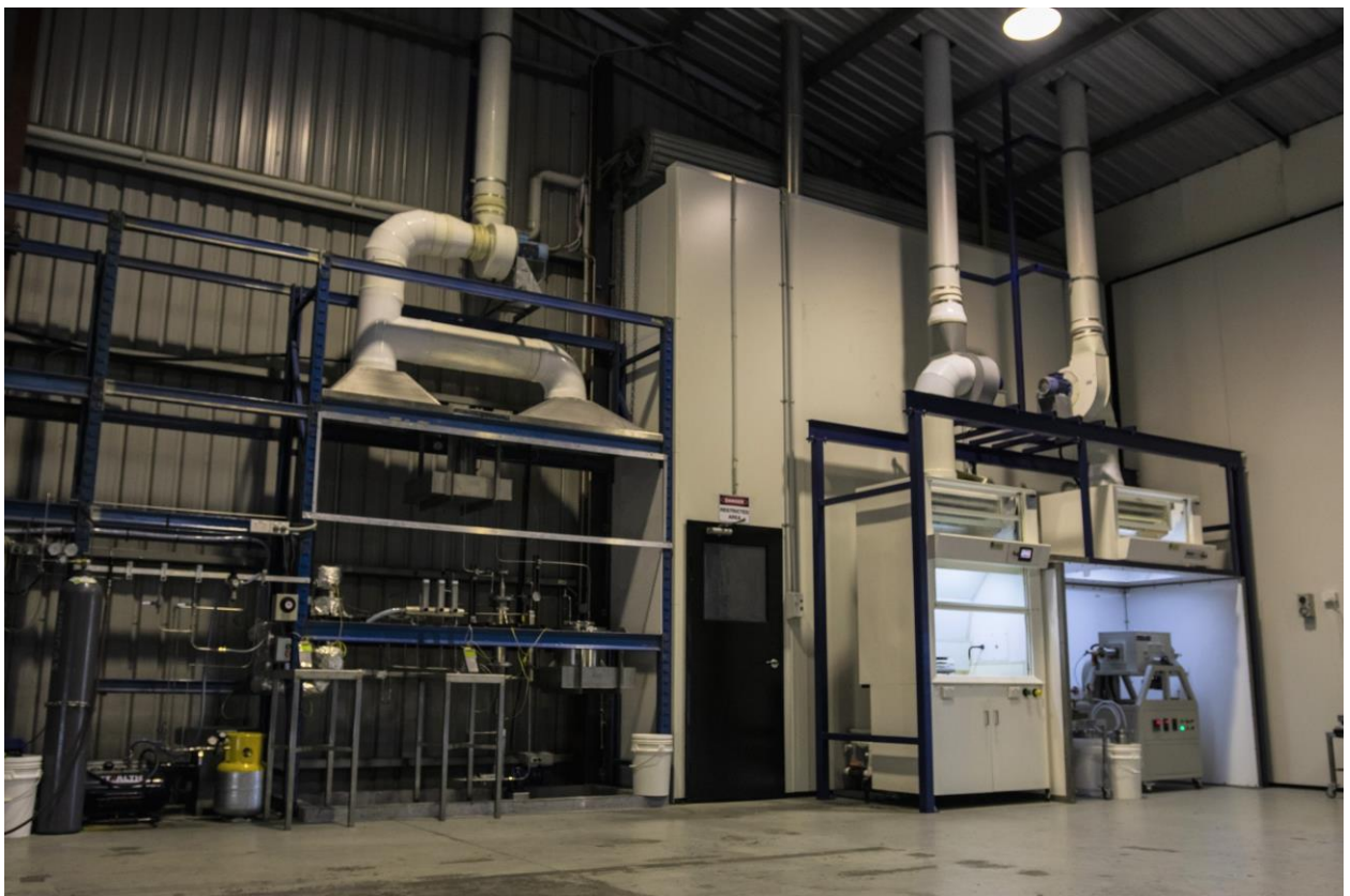
Figure 5: Section of the Alcore Technology Centre upgraded to allow the operation of three new laboratory reactors
