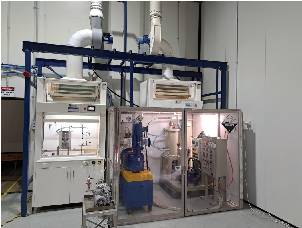
Figure 2: Bath pilot batch reactor (centre) installed at ALCORE Technology Centre
