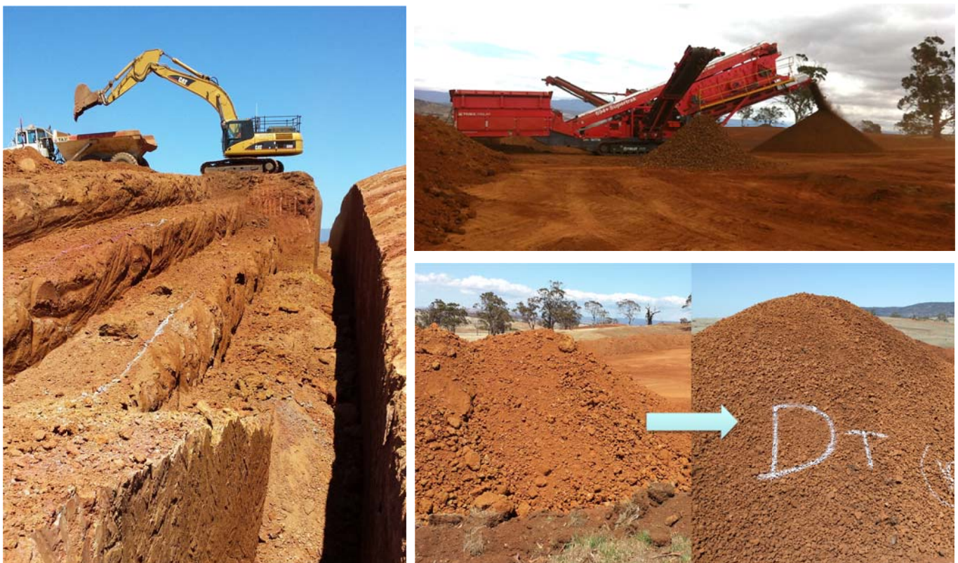
Figure 4: Bald Hill Bauxite Project Mine: Initial slot cut through bauxite formation & Screening ore (left) into product (right)
