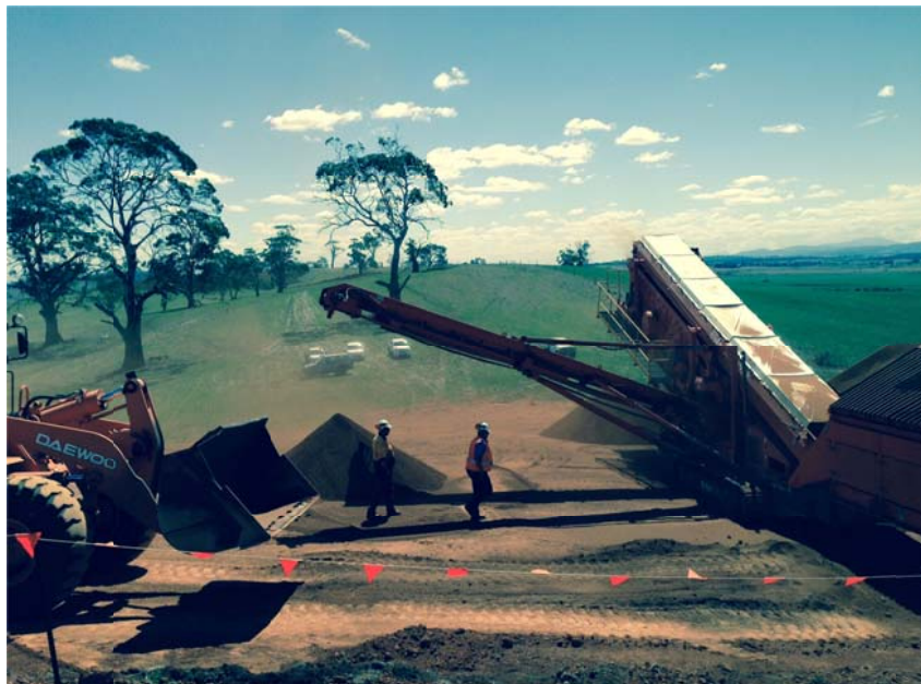
Figure 5: Bald Hill Bauxite Project Mobile Screening Plant. The bauxite forms the barren ridge top extending into the distance
