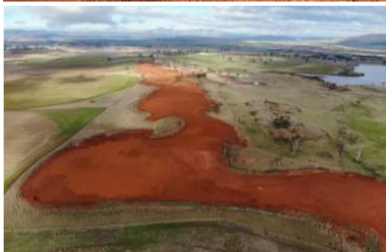
Figure 6 Rehabilitation at Bald Hill mine was nearing completion at the end of the quarter.
