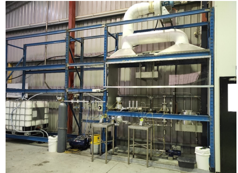
Oleum production plant
