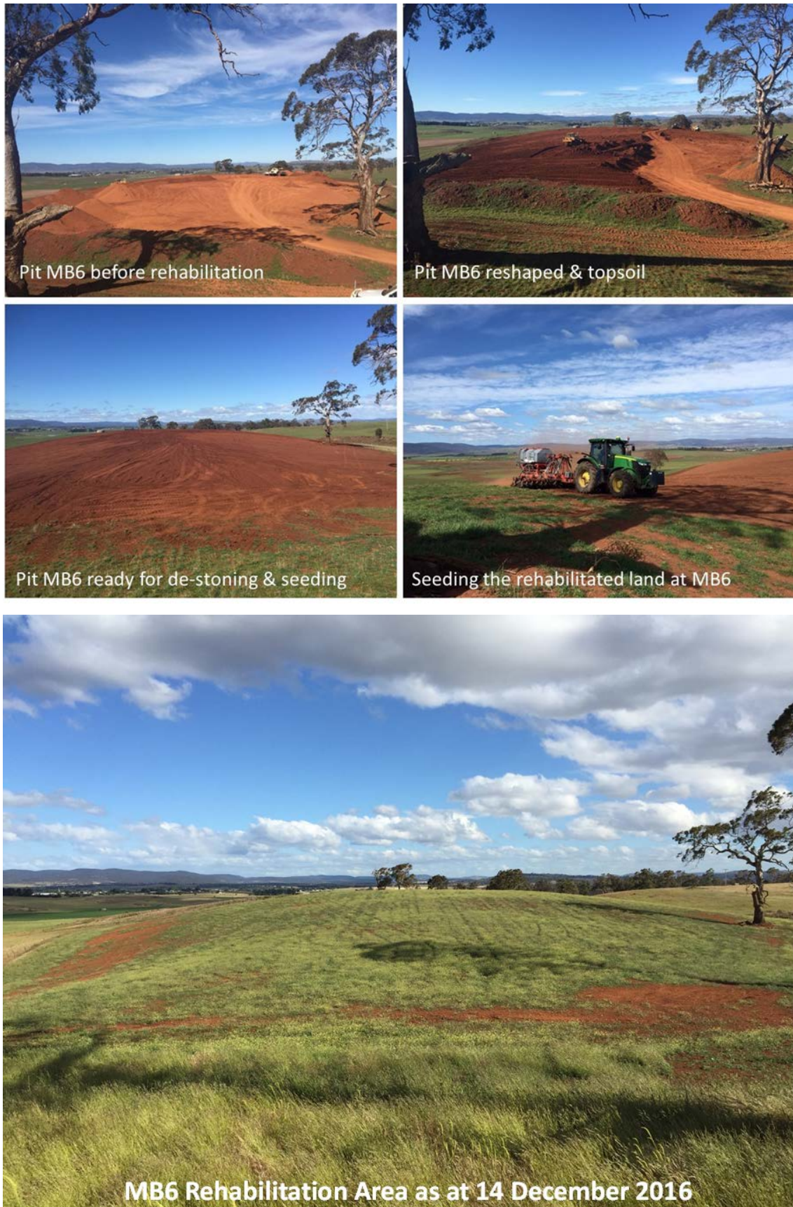
Figure 4: photographic record of rehabilitation processes, with Pit MB6 as the case study
